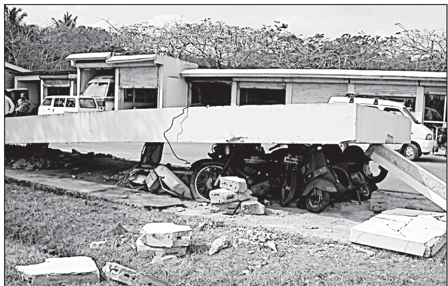
Fig 5 Collapse of a reinforced concrete scooter stand at Port Management Board office in Port Blair (Photo: Hemant Kaushik)
