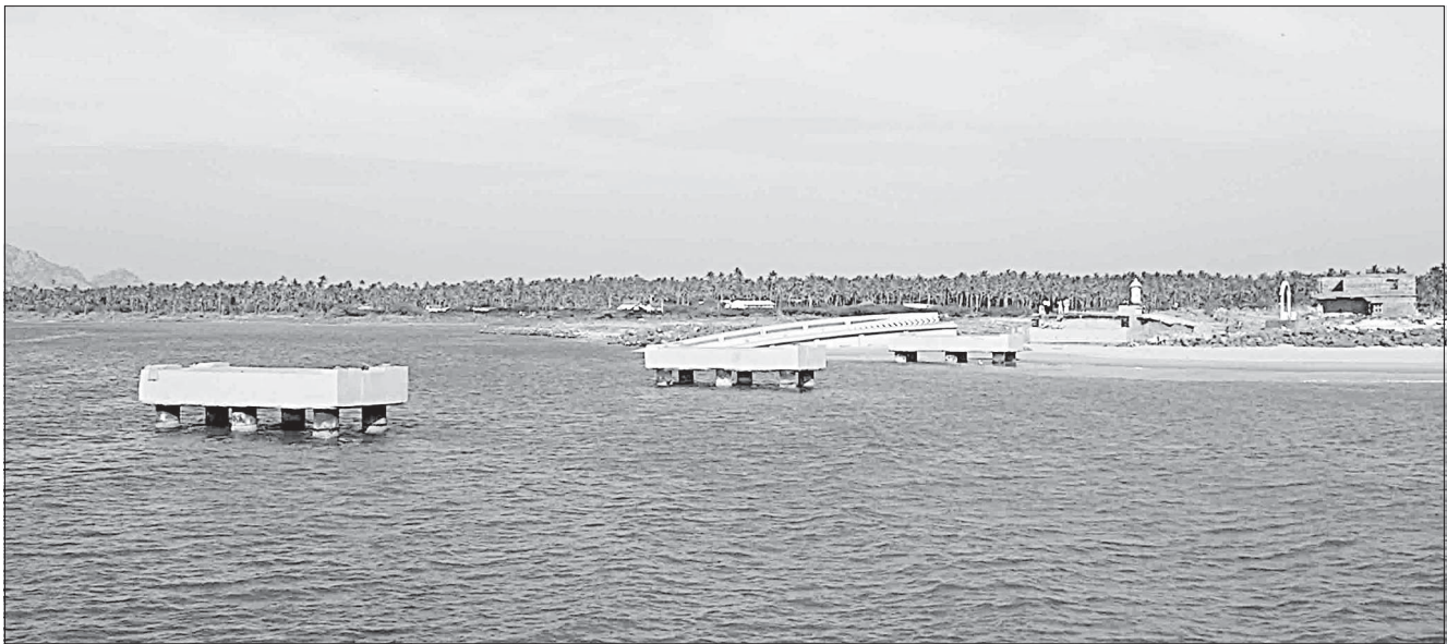
Fig 10 Complete loss of the four span of a RC bridge at Melmannakudi (Photo: Alpa Sheth)
