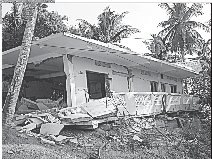
Fig 4 Collapse of a stilt plus one-storey house in reinforced concrete near Port Blair (Photo: Hemant Kaushik)
