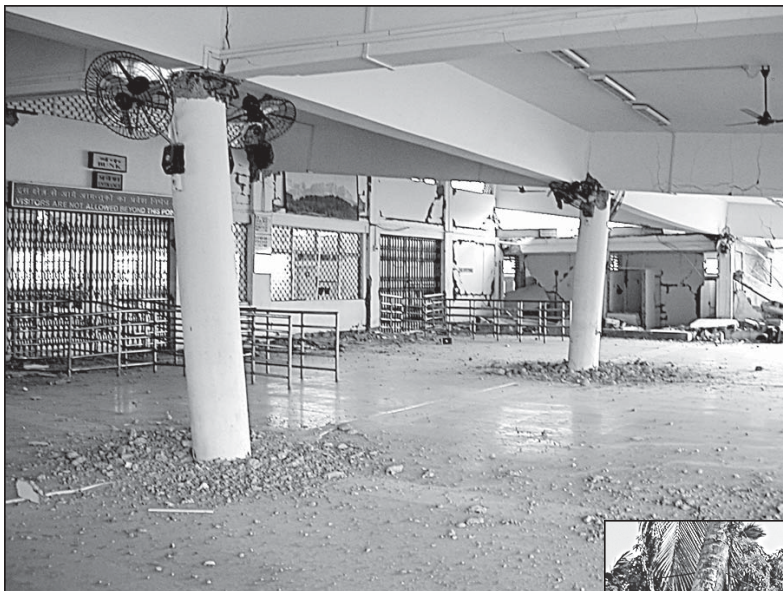
Fig 2 Severe damage to Passenger Terminal Building at Port Blair (Photo: Sudhir K Jain)
