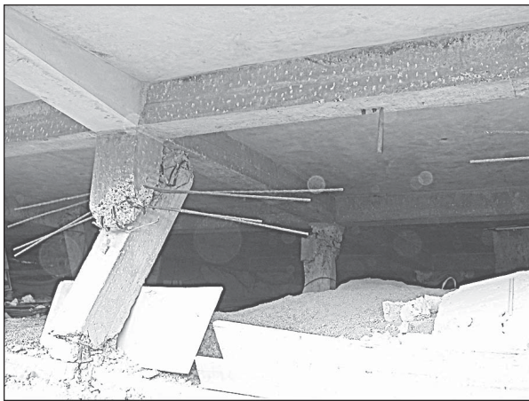
Fig 6 Collapse of three-storey reinforced concrete frame building at Port Blair (Photo: Sudhir K Jain)
