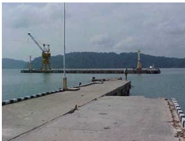
Figure 5. Collapse of the 80 m segment of approach in Great Nicobar Island jetty at Campbell Bay. This has adversely affected the relief work. (Photo: C. V. R. Murty).
