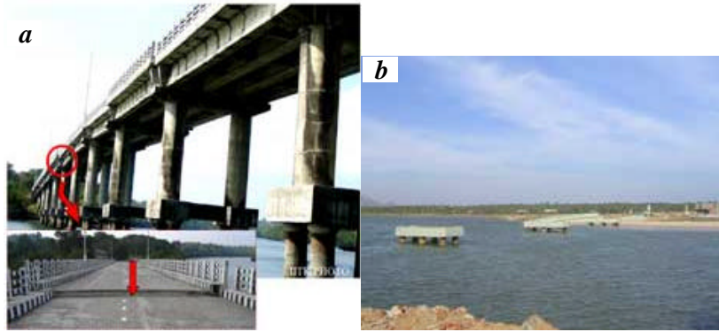
Figure 6. a , Three middle spans of Chengappa Bridge over Austen Strait connecting Middle Andaman and North Andaman Islands, 230 km north of Port Blair fell off from the bearing due to ground shaking. (Photo: Durgesh C. Rai). b , Complete loss of spans of the four-span RC bridge at Melmannakudi due to tsunami. (Photo: Alpa Sheth).
