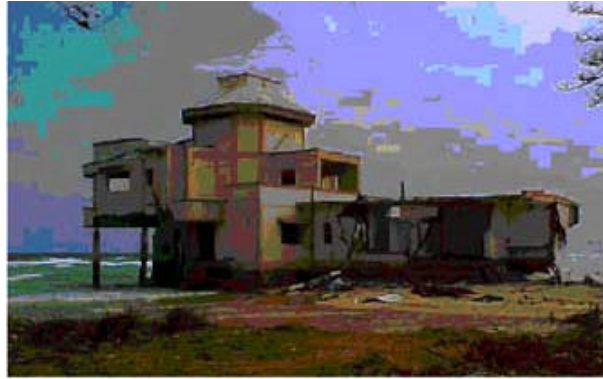
Figure 3. RC frame building (MES Inspection Bungalow) now stands in waters at the Military Residential Colony south of Malacca on the east coast of Car Nicobar Island. (Photo: C. V. R. Murty).
